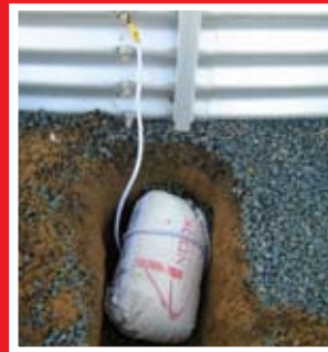
Sacrificial Magnesium Anodes for Corrosion Protection
